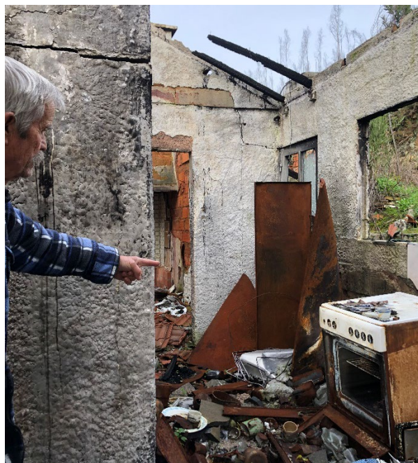
Community member in his destroyed house ©CVP
